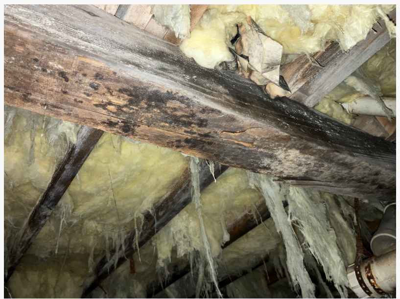
Moisture Damage / Fungi under a home
