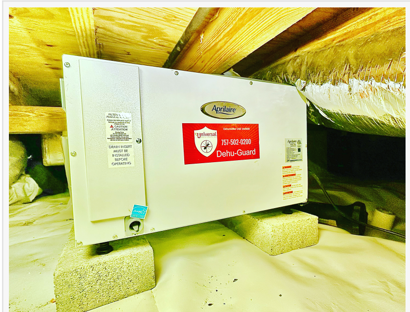
Dehumidifier by Universal Pest & Termite
