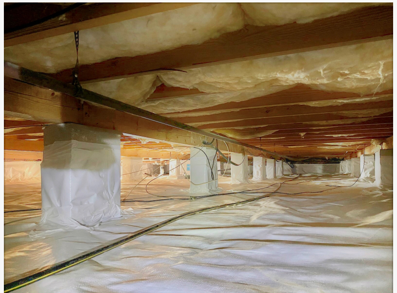
Encapsulation Under Home in Crawl Space
