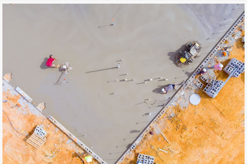
Workers smooth and level a concrete foundation using a concrete polishing machine to ensure a flat and even surface.
