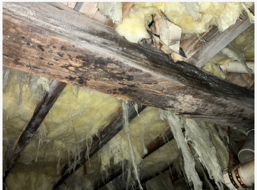
Moisture Damage / Fungi under a home
