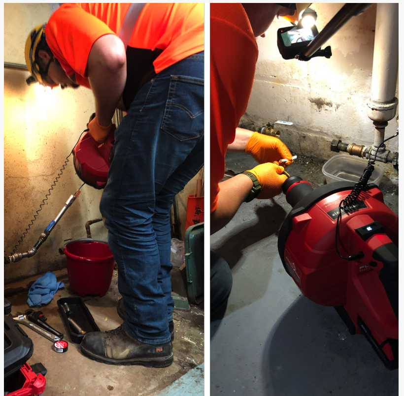
Basement water service line inspections are typical for most New York properties.
