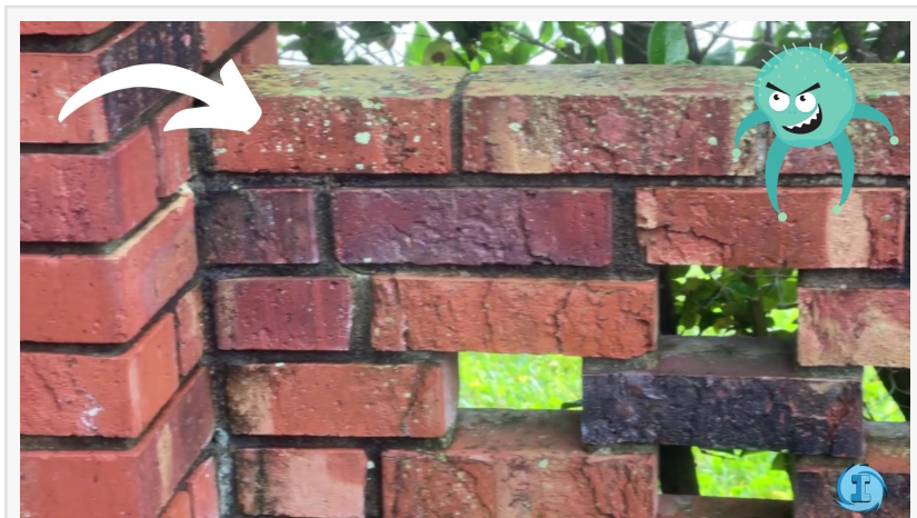
Mold Damage on Fence
