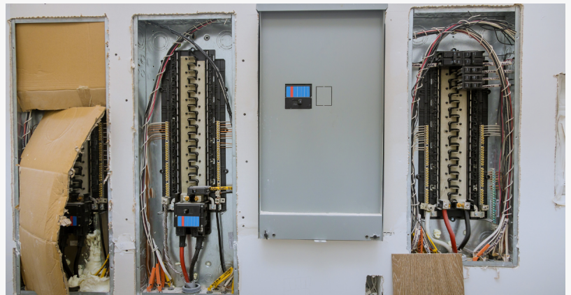
Electrical Panel Services
