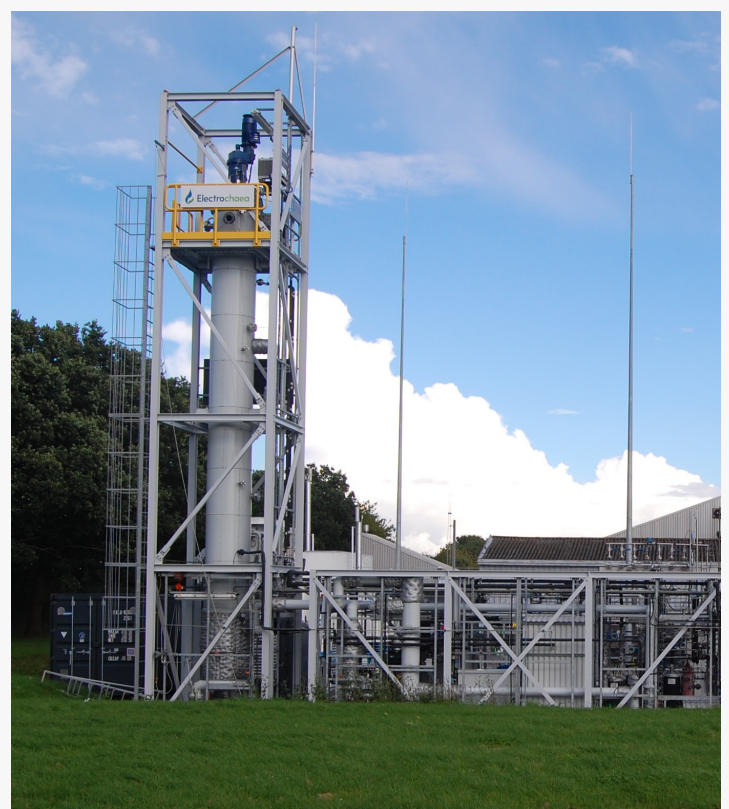
Electrochaea's bioreactor at a pilot plant in Denmark ©Electrochaea
