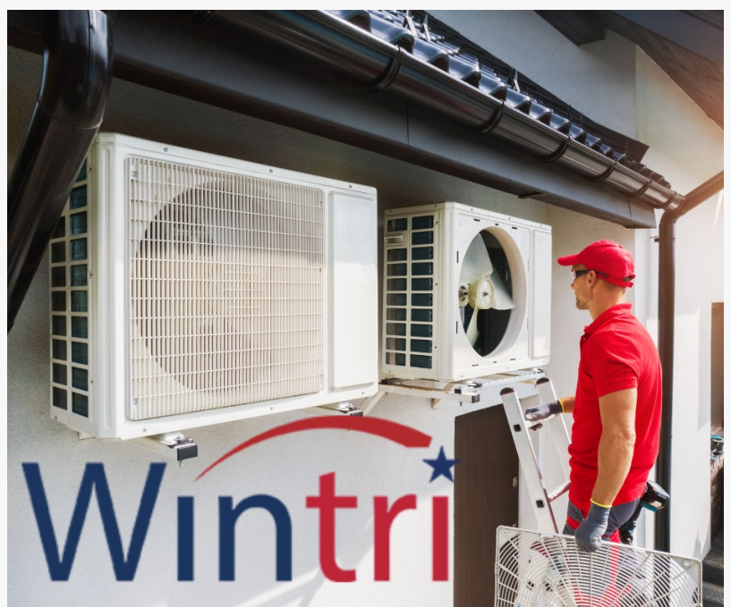
Free HVAC Diagnostic Services
