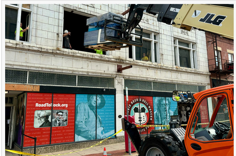
Telehandler loading custom cabinetry from the Rick's Picks exhibit through a second floor window.
