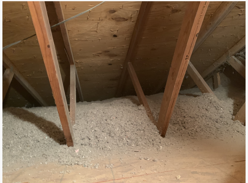
Blown Insulation in an attic
