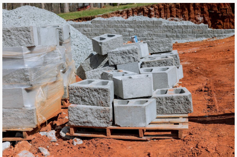
Various concrete materials neatly arranged on a bare construction site, awaiting the start of the project.
