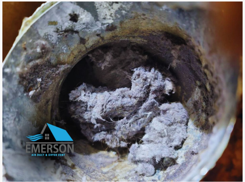
Air Duct Before Cleaning by Emerson Pro Services
