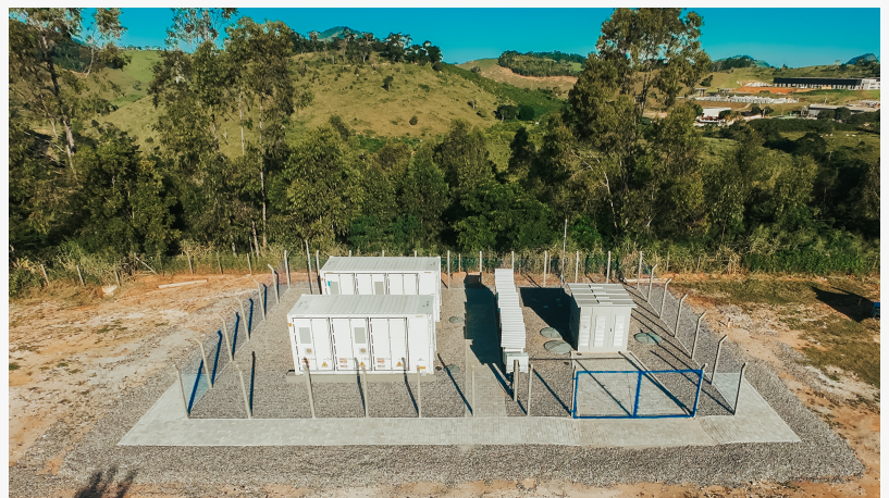
Photo of a Battery Energy Storage System (BESS) installed at Cofril, one of Matrix Energia's clients, supporting efficient energy management and sustainability goals.
