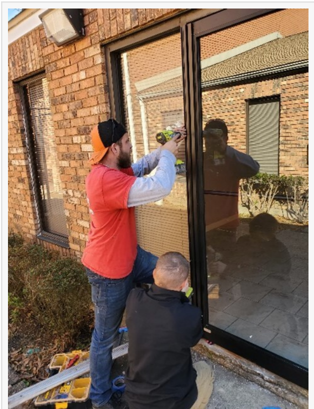
AA Screens & Glass Technicians install custom glass windows in a local Gretna home.
