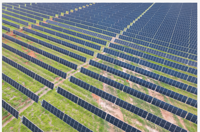
Atlas Renewable Energy's Boa Sorte Solar Plant (438 MWp) located in Minas Gerais, Brazil.
