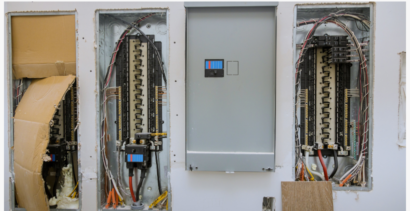
Electrical Panel Services
