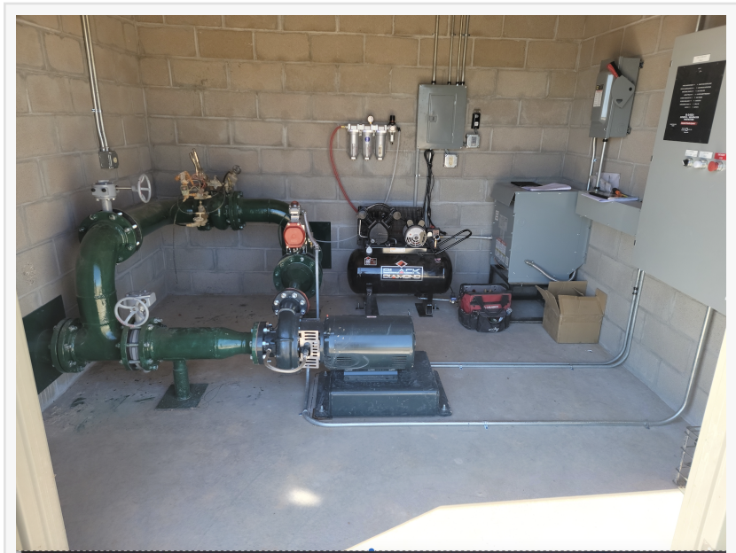
Rentricity REAP Turbine & Control Configuration
