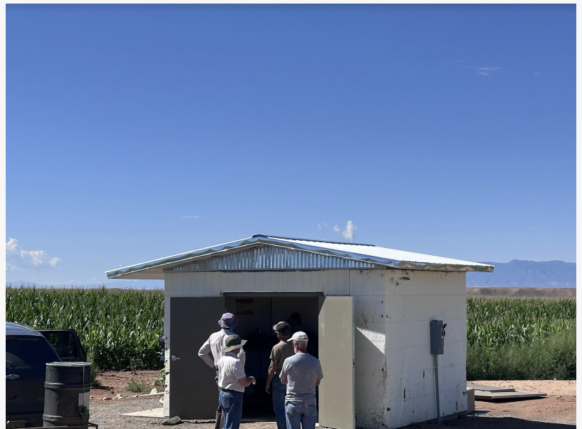
Ute Tribe Farm & Ranch Enterprise REAP Powerhouse
