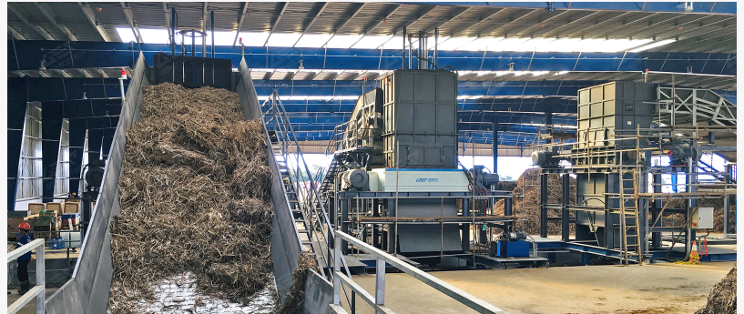
Biomass Fuel Supply System
