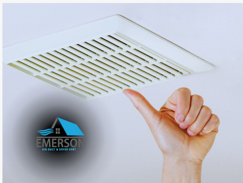
Air Duct Maintenance by Emerson Pro Services
