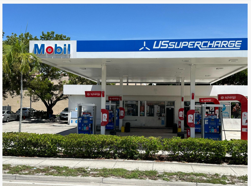
Victoria Park Mobil Station's new up to 240 Kw Supercharger 606 N. Federal Hwy.
