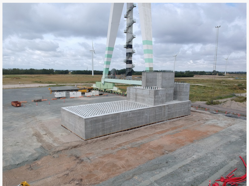
Completed: the 3,700 metric ton foundation for the new test bench for main bearing for wind turbines up to 25MW
