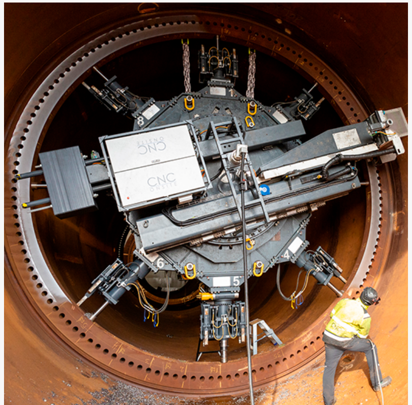
The Goliath precision machine from CNC Onsite can mill large diameter offshore flanges of up to 10-meter
