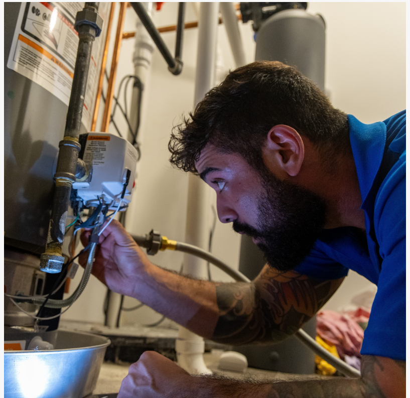
A J. Blanton Plumbing technician fixing a water heater, part of the Free Annual Home Winterization service offered to No Drip Club members in Chicago.
