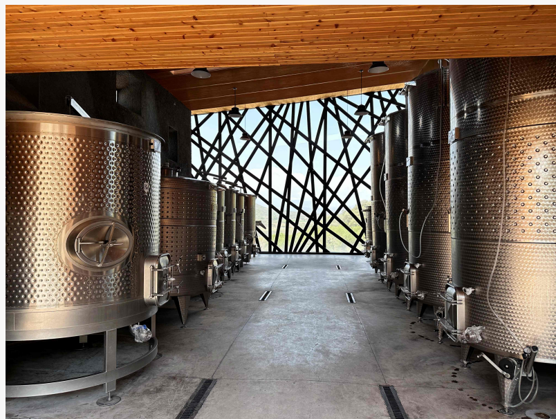
Stainless steel wine tanks at Puerta del Lobo Winery with a view of the El Lobo Valley in Querétaro, Mexico
