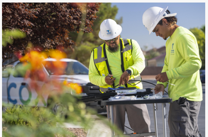
Contractors install fiber on behalf of Cox in a southwest Las Vegas neighborhood
