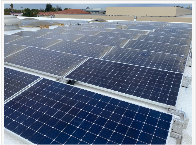
Synergy 768 Commercial Solar
