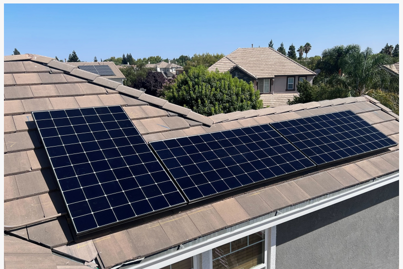
Synergy 768 Residential Installation
