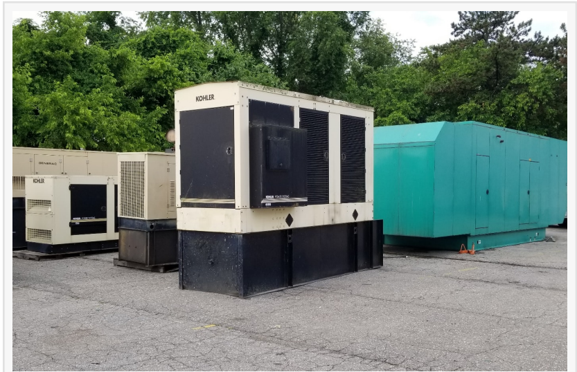
Backup Power Market Insights
