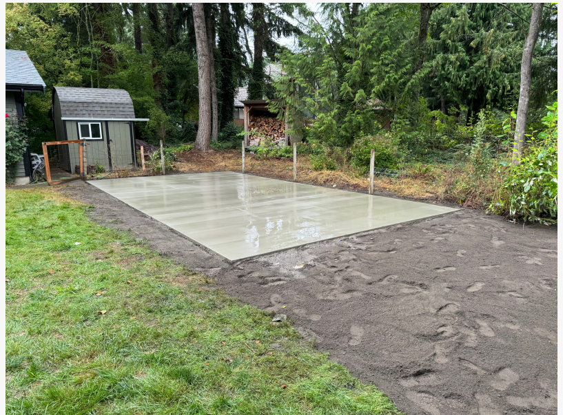
Concrete Paver for Hot Tub
