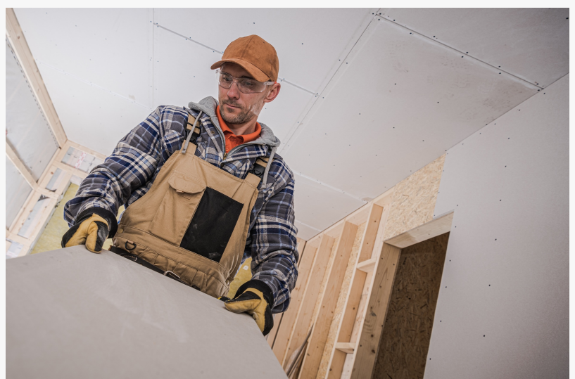
A man repairs drywall after water damage affects a home
