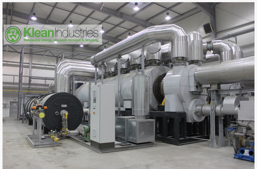
Klean Industries - End-of-Life Tyre Pyrolysis & Tire Recycling Recycling System
