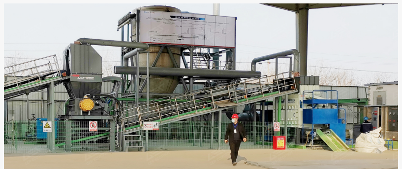
Fiber-Reinforced Plastic Processing Plant
