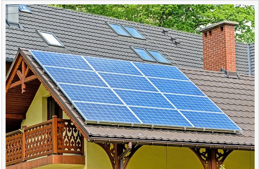
Federal Tax Credit for Solar Panels
