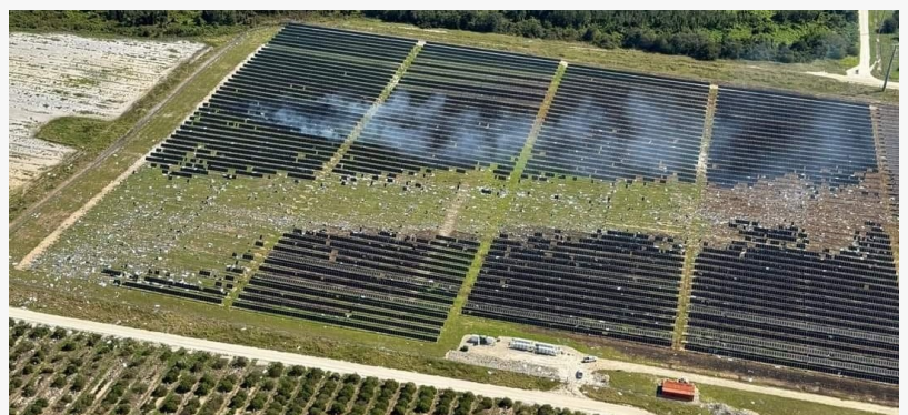
Image Source: Duke Energy (Florida solar panel field hurricane damage)
