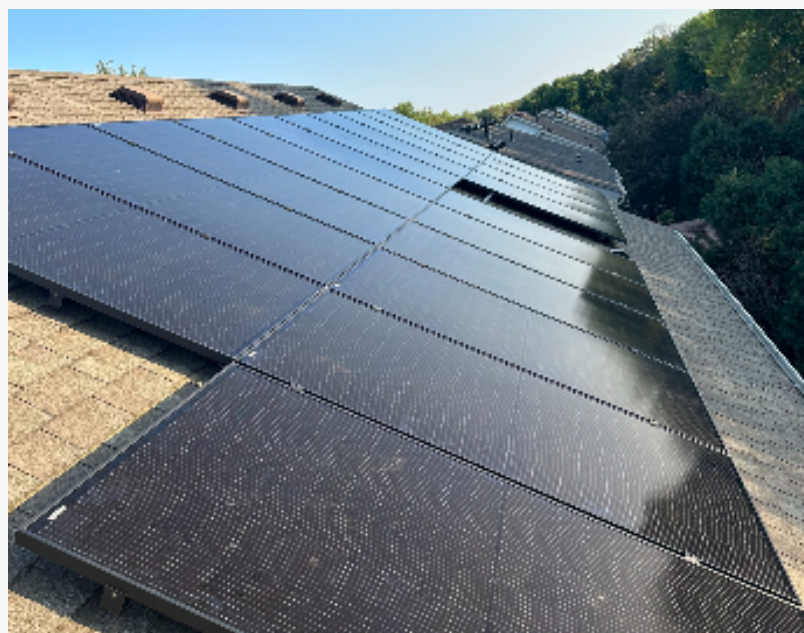
Wolf River Solar Installation
