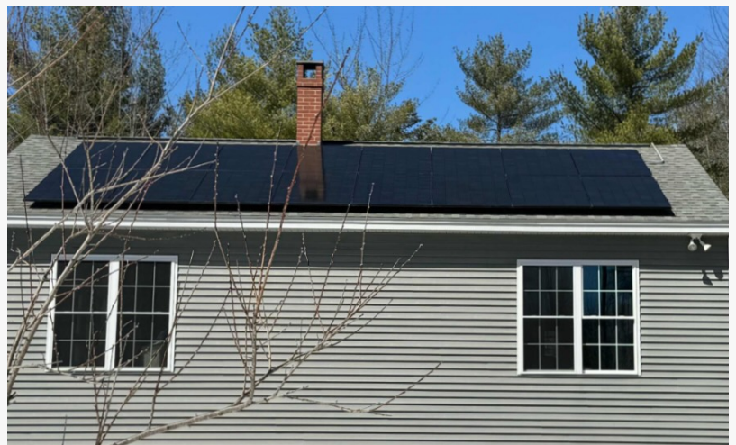
Suncovia Residential Solar Installation
