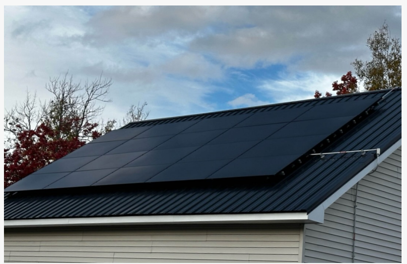
Suncovia Rooftop Solar Installation
