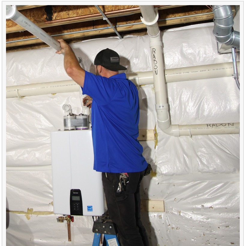
A J. Blanton Plumbing technician installs a continuous water heater, providing reliable plumbing repair and emergency plumbing services in support of the Park District of Highland Park's Winter Wonderland Event 2024.
