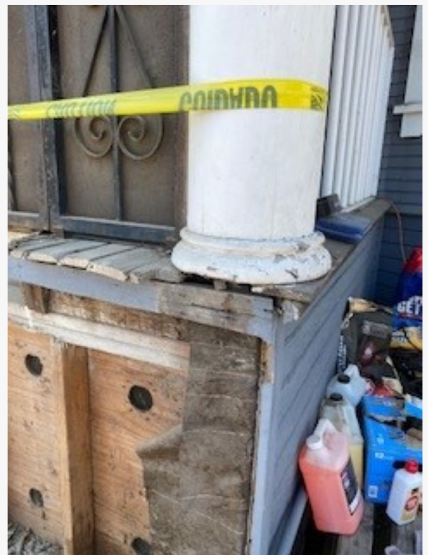
Home Damage Fireworks explosion
