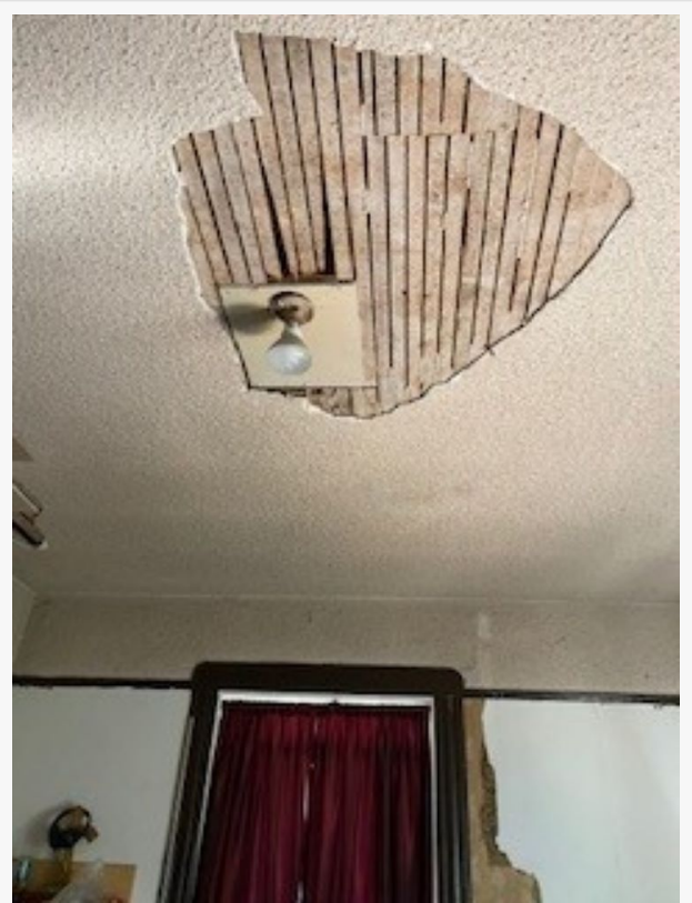
Ceilin Damage- LA City Fireworks Damage
