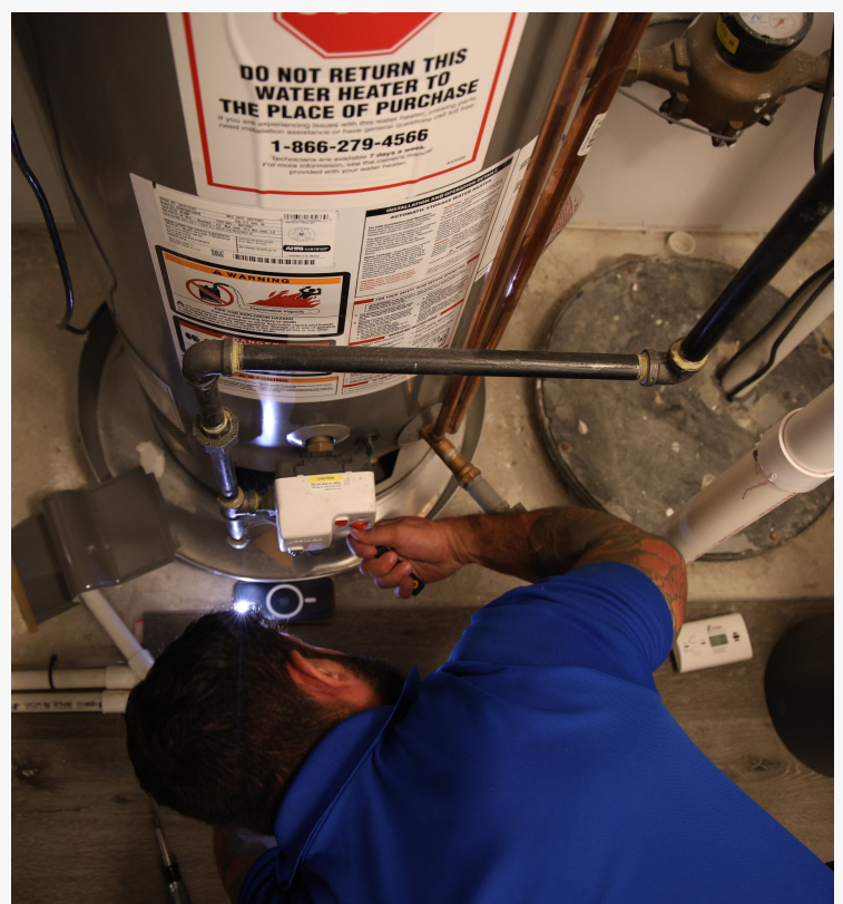
A J. Blanton Plumbing technician at work, highlighting the company's expanded services in Skokie, including water heater maintenance, skilled plumbing contractors, and expert water heater installation.
