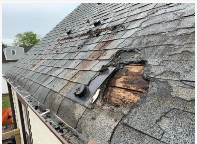
Damaged roof under improperly installed solar panels
