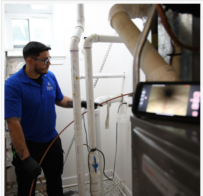
A J. Blanton Plumbing technician conducts a drain camera inspection, showcasing the company's expertise in water heater services and gas line installations as part of their membership in the Rogers Park Business Alliance.
