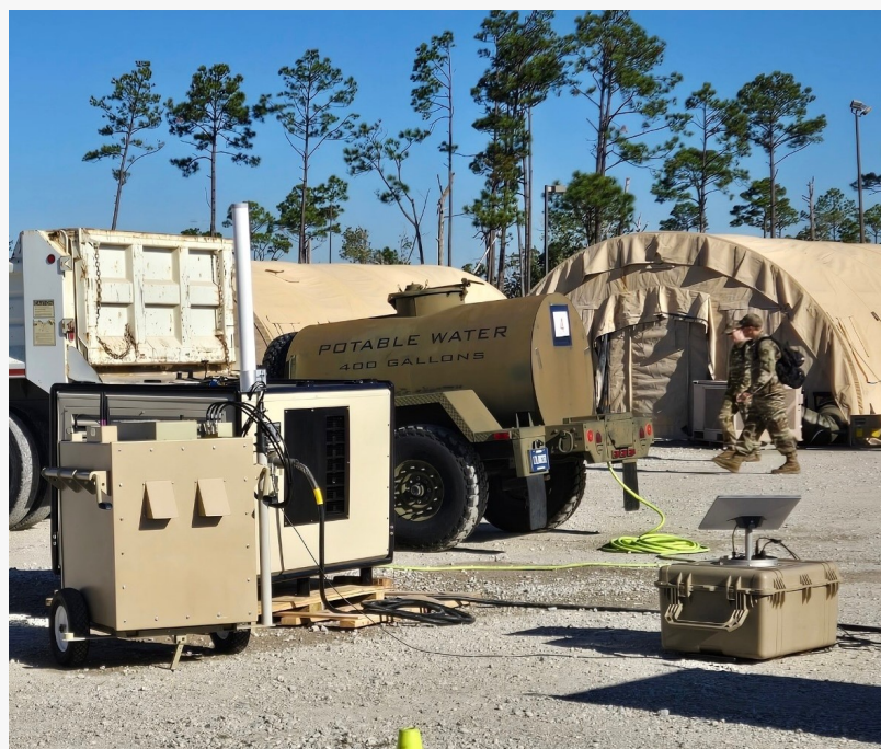
Genesis Systems' WaterCube and SEMPRES's 5G Network in Operation at Tyndall AFB
