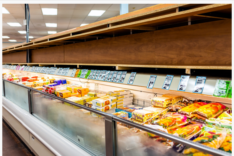
Open air refrigeration in a grocery store
