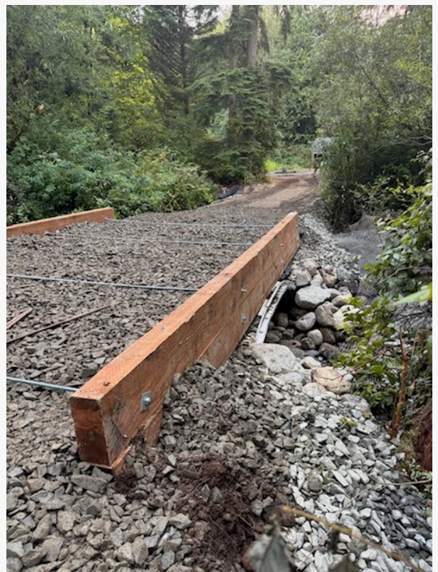
Gravel Installation and Excavation Job in North Seattle Washington with Indepth Excavation
