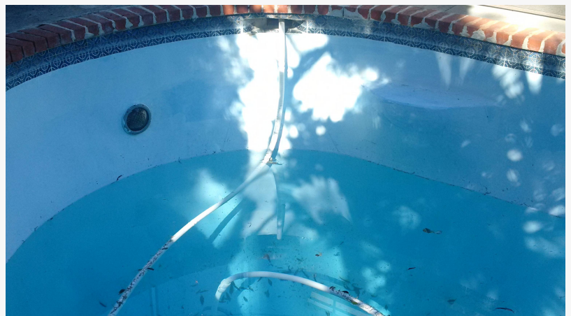
Empty Pool From A Pool Leak
