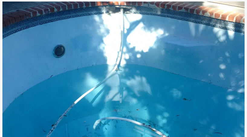
A swimming pool experiencing a water loss from a pool leak.
