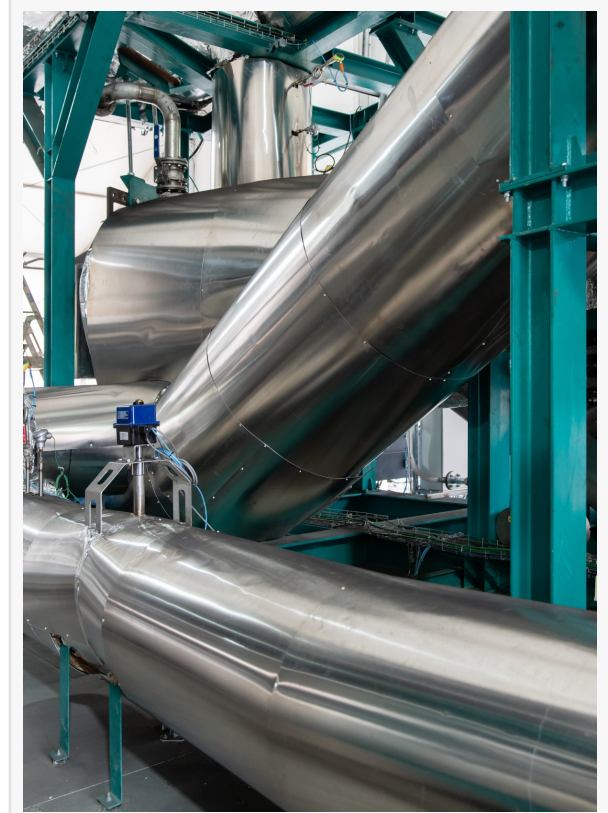
Part of the thermolysis module that converts residual biomass and organic waste into renewable gas and biocarbon (or biochar).
