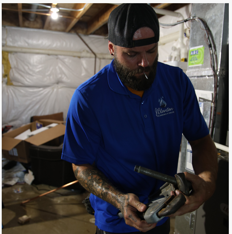
A J. Blanton Plumbing technician installs a residential water heater, showcasing the company's expert water heater installation services and skilled plumbing contractors in support of the Naperville Park District's Santa's Workshop 2024.
