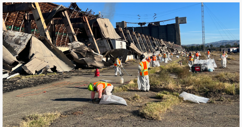
ATI technicians removing debris after the Tustin North Hangar fire
