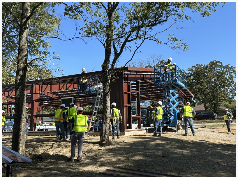
The Mueller Team work to finish the Women's Crisis Services new building.
