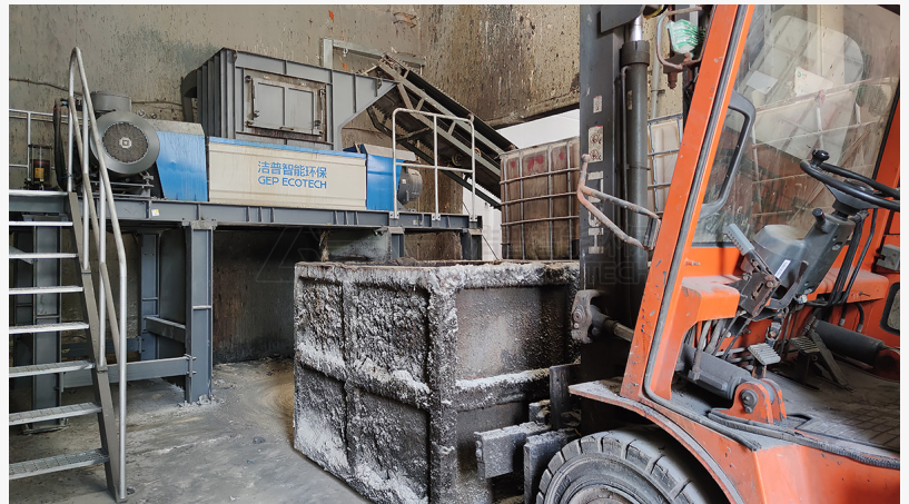
Hazardous Waste Shredder
